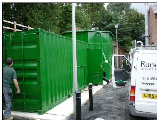
FIGURE 14 A CONTAINERISED WOOD CHIP HEATING SYSTEM AT A DEFRA OFFICE
